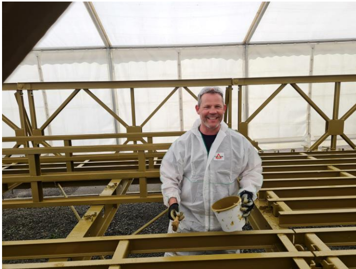
A Fenland Sapper refurbishing the Bailey Bridge in the Pegasus Bridge Museum
